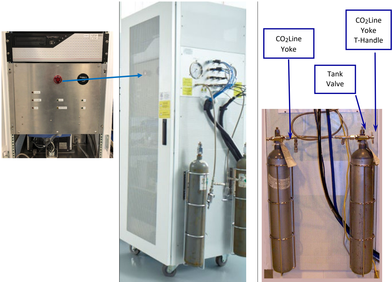
Figure 7.2 Emergency Stop and Electronics Rack with mounted CO 2 Tanks
